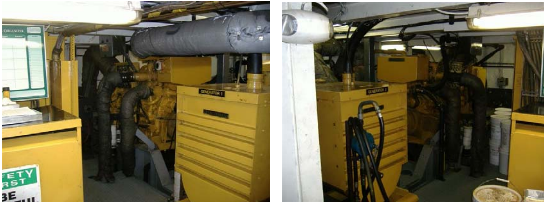
Figure 1: Auxiliary Genset Arrangement
